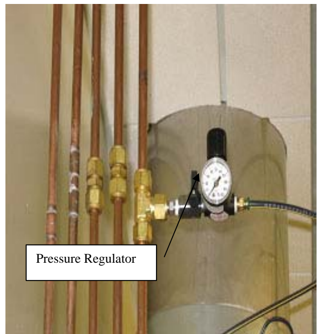
FIGURE 4. PRESSURE REGULATOR AND TYPICAL TIE IN TO EXISTING AIR LINES ON TOP OF EACH FUME HOOD WITH TO ACTIVATE CABLE/PULLEY SYSTEM SHOWN IN FIGURE 3.
