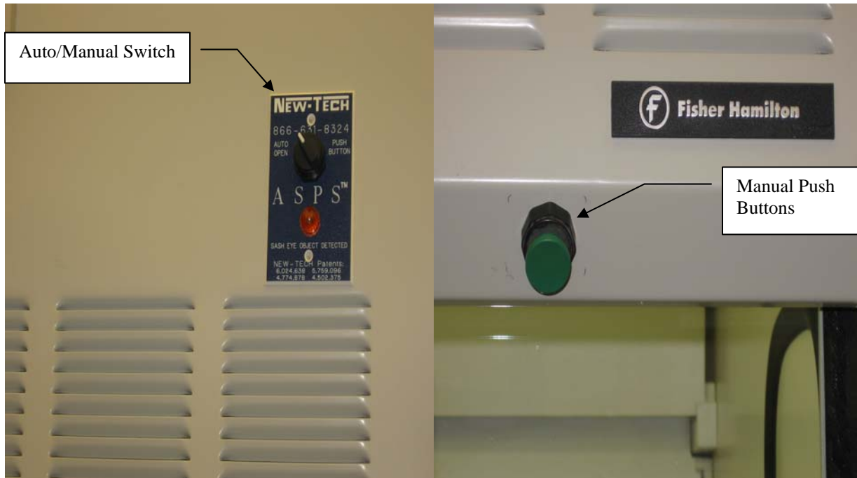
FIGURE 2. A USER CAN SWITCH TO MANUAL MODE AND USE THE PUSH BUTTONS TO RAISE AND LOWER THE FUME HOOD SASH.
