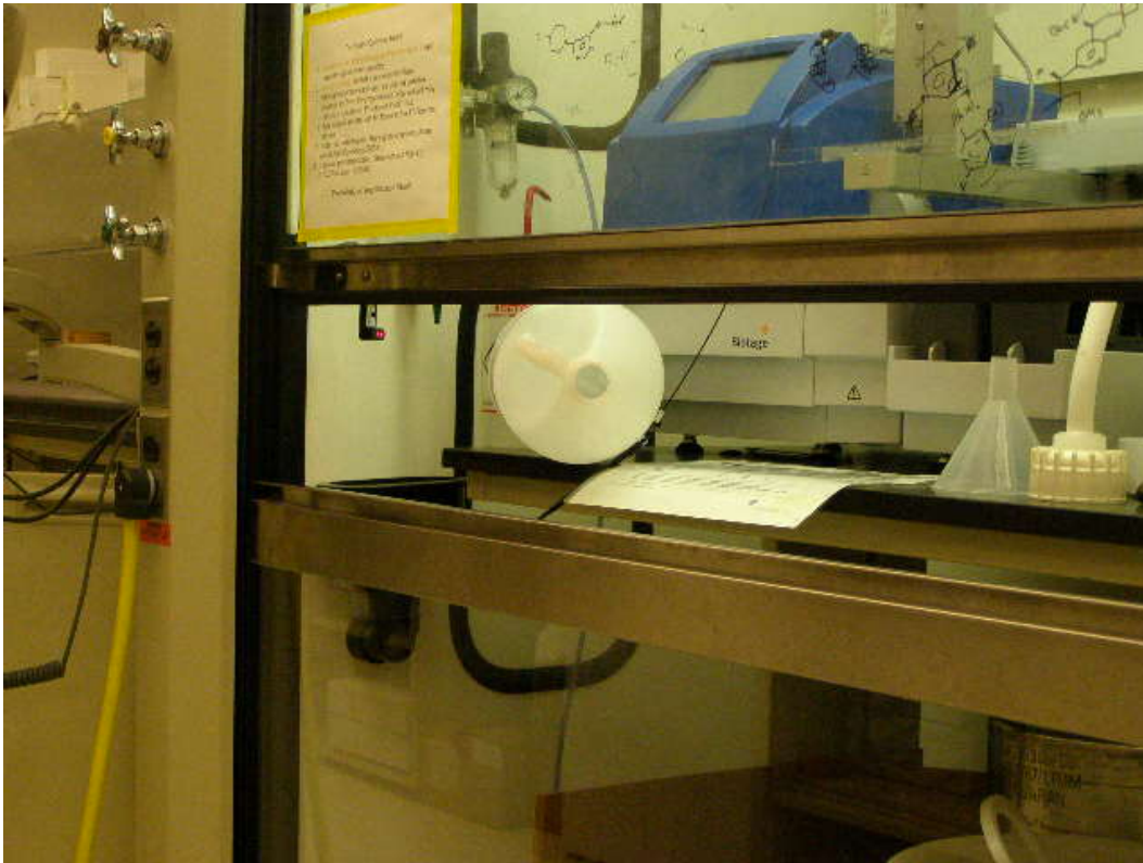
FIGURE A-5. ASPCS HOOD 4150.6 WITH EMPTY BOTTLE OBSTRUCTION CAUSING EXCESSIVE EXHAUST USAGE.
