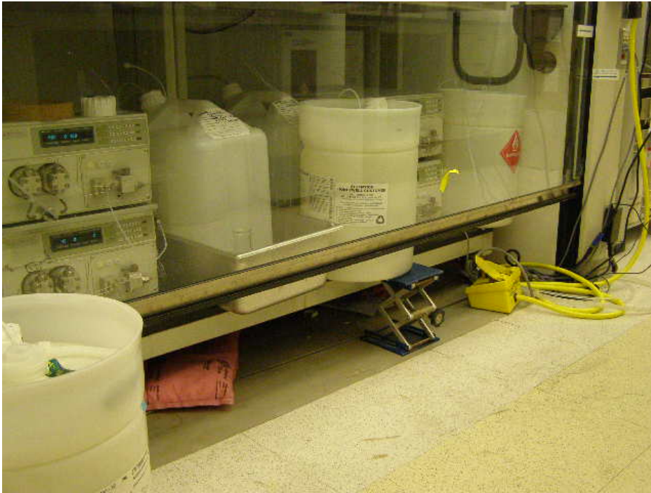
FIGURE 19. CHEMICAL BUCKETS AND OTHER OBSTRUCTIONS KEEP LOWER LIMIT SWITCH FROM MAKING CONTACT
