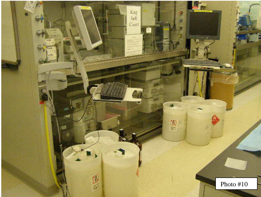
FIGURE 20. CORRECTING OBSTRUCTIONS BY LENGTHENING HOSES AND MOVING CHEMICAL BUCKETS OUTSIDE LOWER SASH. ASPCS CAN NOW WORK PROPERLY WITHOUT USER ASSISTANCE.
